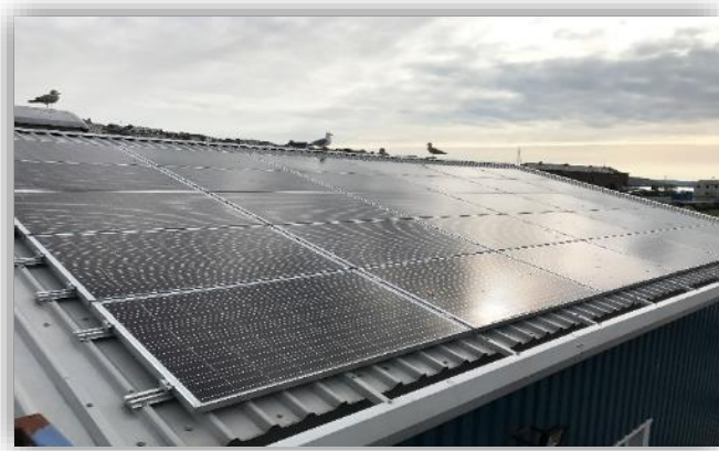
Solar panel with 50 Kw capacity
