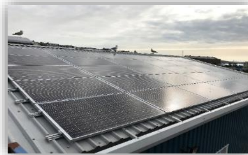
Solar panel with 50 Kw capacity
